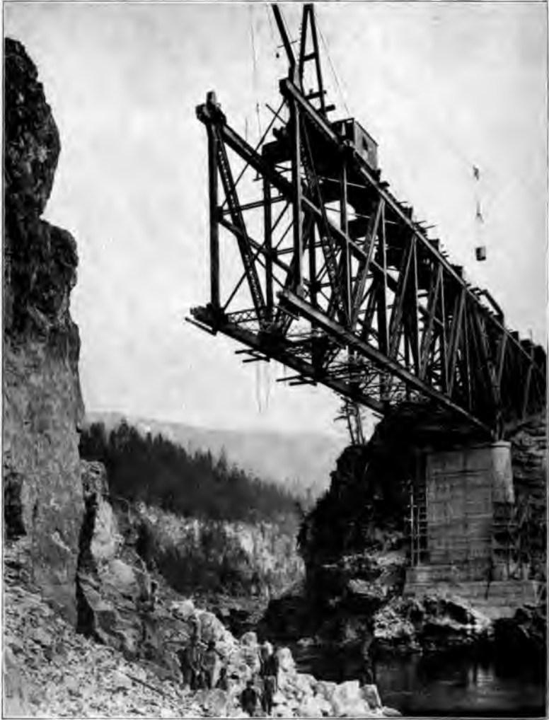
BUILDING THE WONDERFUL BRIDGE OF THE IDAHO & WASHINGTON NORTHERN OVER THE PEND OREILLE RIVER, WASHINGTON
